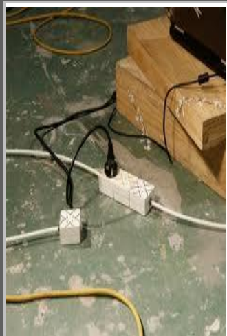
Extension cords on floor; trip hazard
