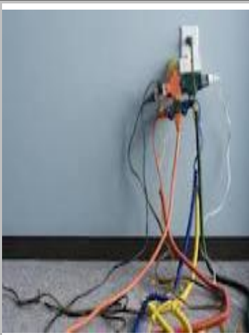
Too many plugged into one outlet
