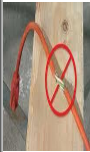
Insulation Missing; Exposed wires
